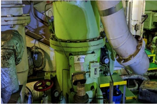
Gambar 3. Filter Lubricating Oil
