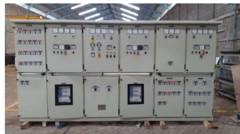
Gambar 1. Main Switch Board
