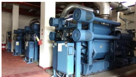
Gambar 7. Generator Set Terminal 1 (PT. Angkasa Pura 1 Juanda, 2017)
